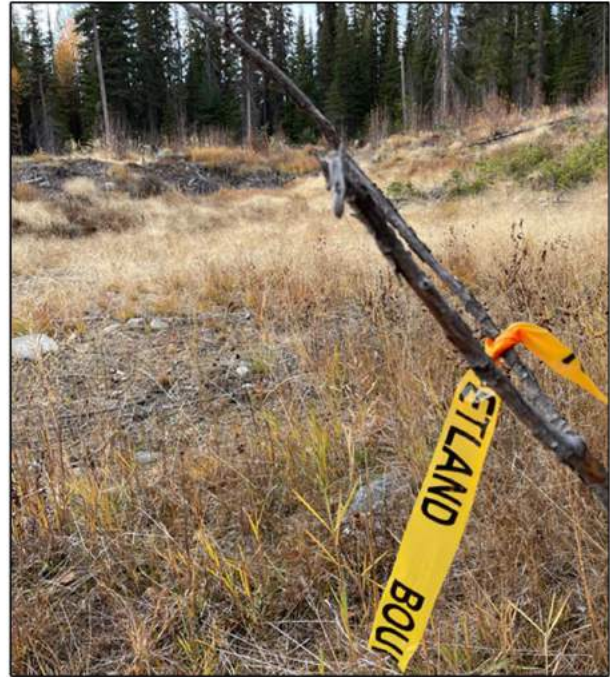
1(b)ii Fireline bulldozed through wetland area, Davis Fire, Montana 2018.
